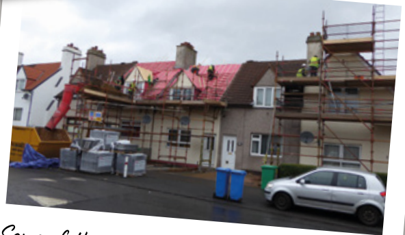
Some of the roofing work undertaken as part of our planned maintenance programme
